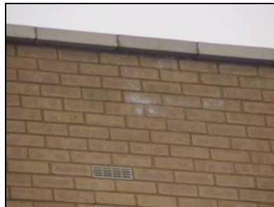
Efflorescence. Also note the weep holes to the lintels above the windows
