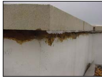
Shows mastic drip has been added
