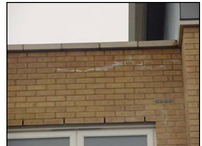
Adjoining properties Efflorescence
