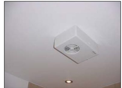
Extract fan Need to identify where the extract fan discharges to
