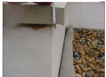
Location of drip next to wall
